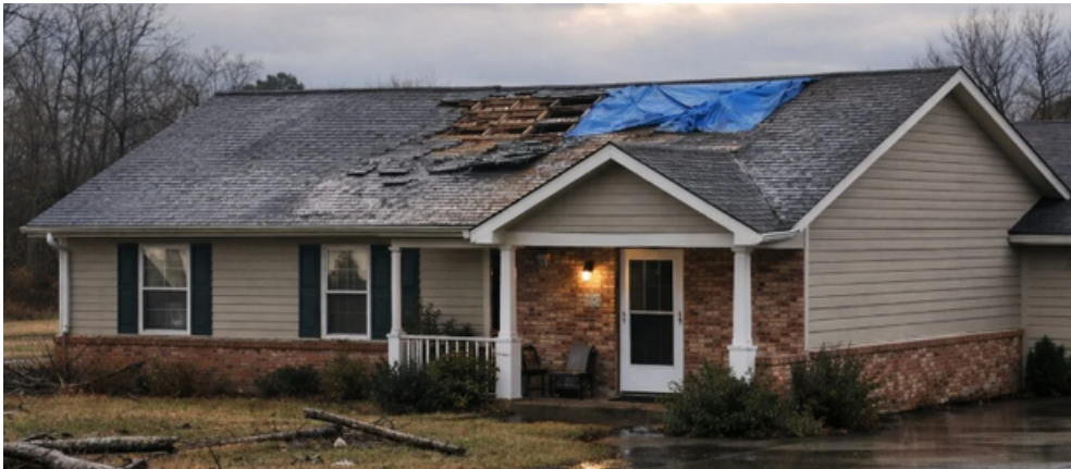
Apparent Defects, Damages, Deficiencies - Roof - Damaged Flashing
